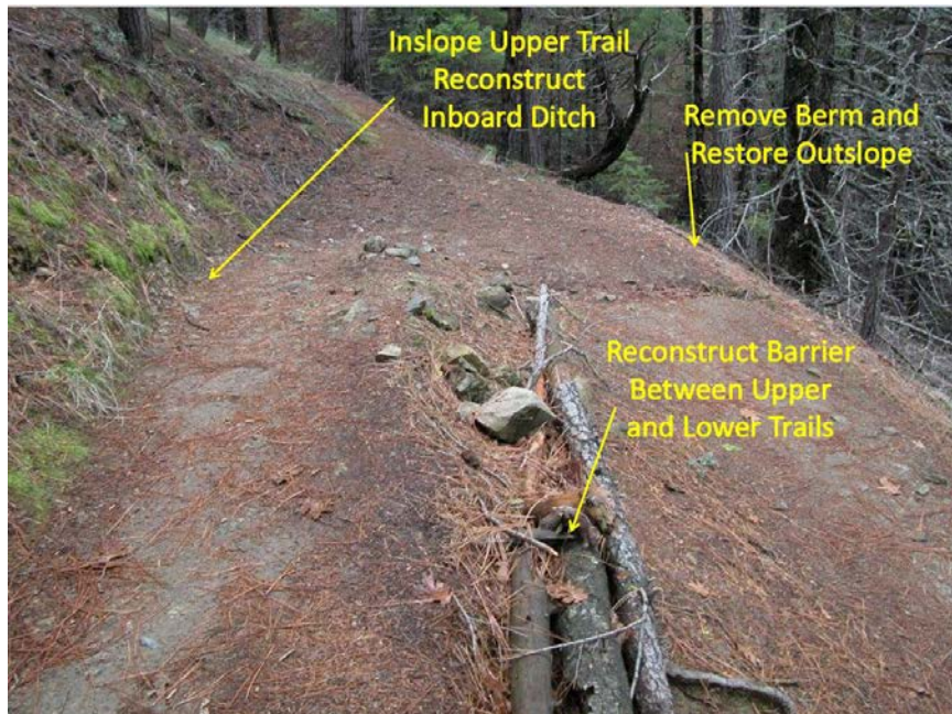
Photo 25.13 - Switchback Requiring Maintenance
