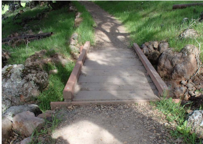
Photo 25.11 - Worn Tread Approach
