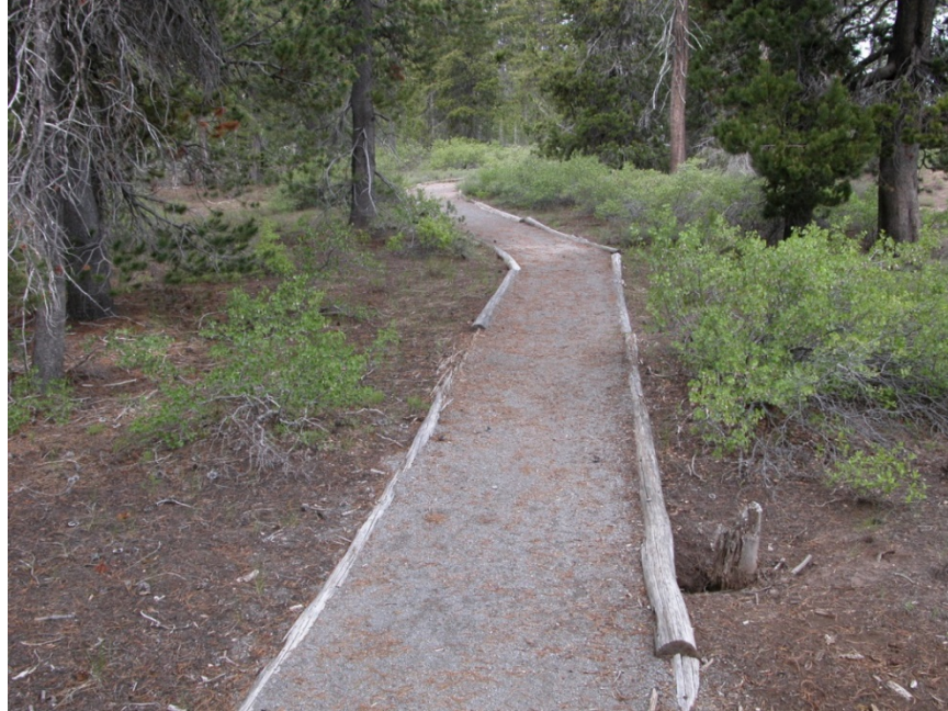
Photo 25.12 - Turnpike Requiring Surface Maintenance
