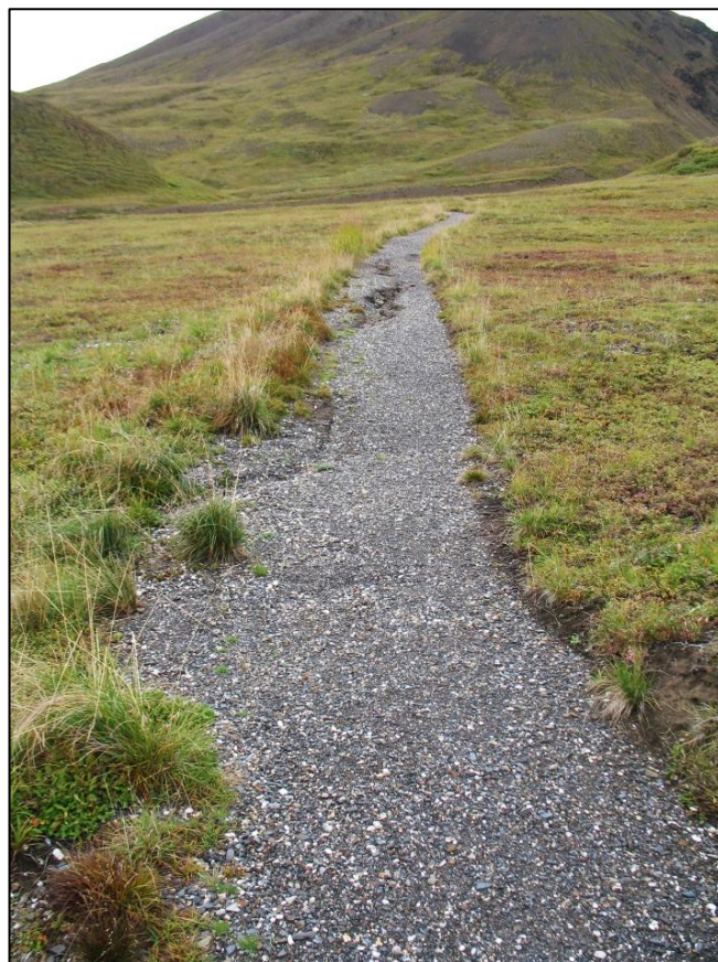
Photo 25.7 - Aggregate Surfacing Requiring Maintenance
