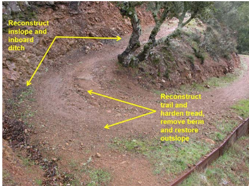
Photo 25.14 - Switchback Requiring Maintenance, continued
